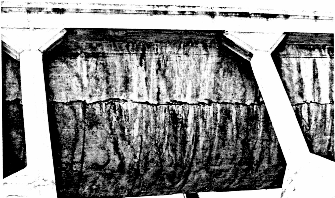
Illustration 21 Shell showing repaired lower section, 1988
